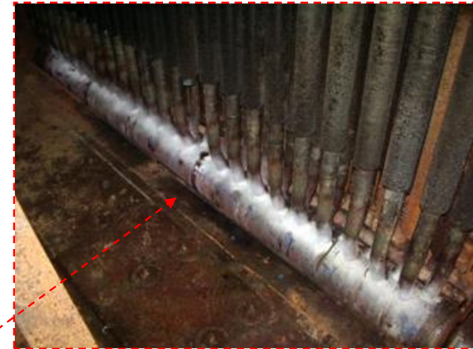
Low cycle fatigue cracks
